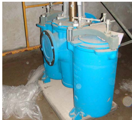
Eaton Filtration duplex strainer (EPA OIG photo)
