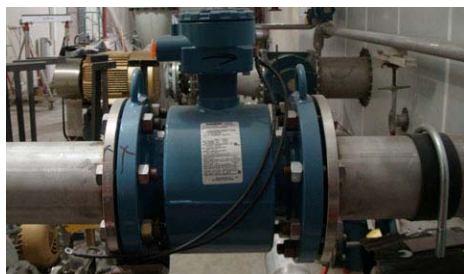
Rosemount magnetic flowtube. (EPA OIG photo)
